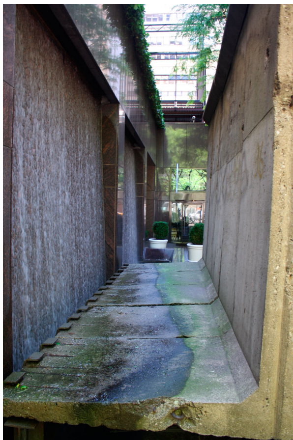
Figure 2 The waterfall that wets the base of the wall, causing biological growth and fully saturating the concrete substrate. Corrosion of rebar and loss of substrate can be seen on the left side of the base. Image: © Kiernan Graves, 2013.
