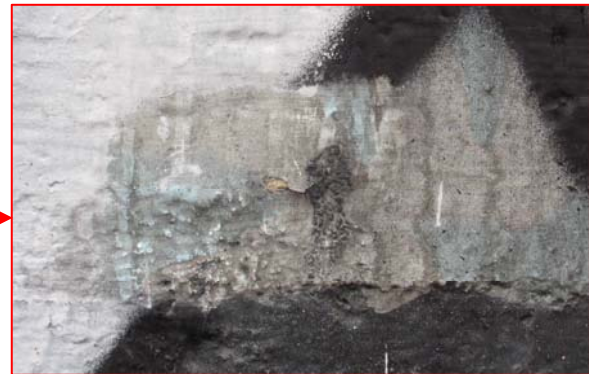
Figure 10.20: Detail; results of cleaning trial 102-T.19 on the more soluble graffiti paint. Photo: Courtauld Institute CWPD 2007
