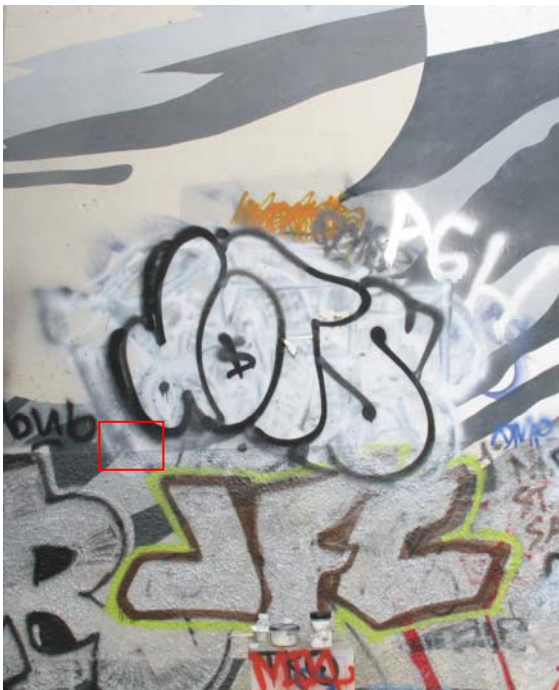
Figure 10.47: The lower third of the mural's support is covered with a highly textured, cement-based surface know as 'stucco'. The heavy texture can make it difficult to achieve a homogeneous result during cleaning. Photo: Courtauld Institute CWPD 2007
