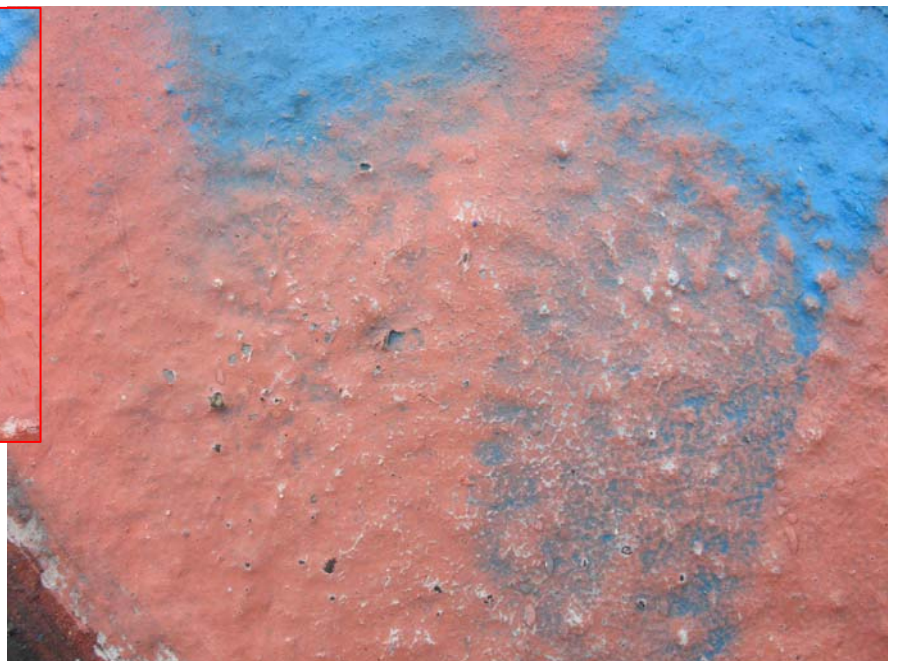
Figure 10.103 (above right): Site of cleaning trial105-T.13, post-cleaning. The proprietary graffiti removal product was unable to successfully remove all aerosol paint and visibly damaged the mural by causing mobilization and cracking of the original paint layer. Photo: Courtauld Institute CWPD 2007
