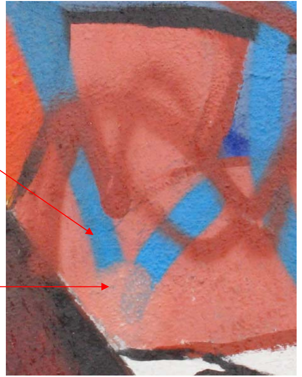
Figure 10.111: Sample locations for the evaluation of cleaning trial 105-T.13. (A) Control sample – uncleaned, no graffiti; (B) Area damaged by cleaning with proprietary graffiti removal product, Mötsenböcker's Lift Off 4®. Photo: Courtauld Institute CWPD 2007
