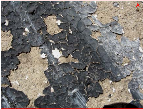
Figure 10.126: Detail; extensive cracking and loss of the original paint layer has exposed the cement support surface and evidence of the white preparatory paint layer applied to the support surface prior to painting. Photo: Courtauld Institute CWPD 2007
